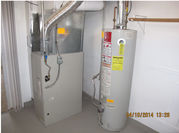
Furnace & Water Heater in Basement
